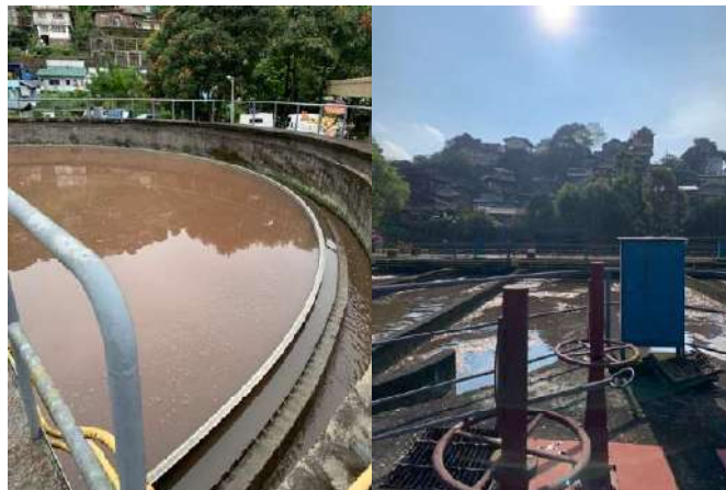
Note. Images of the (left) Primary clarifier and (right) sampling station in BSTP
