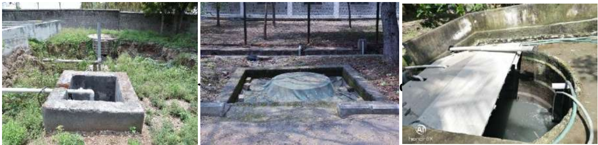
Fig. 9. Water collection and reservoirs tanks.
