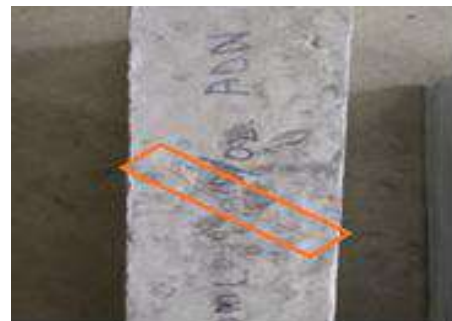
Fig. 3: Initiation of cracks on concrete.
