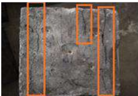
Fig. 2: Initiation of cracks on concrete.
