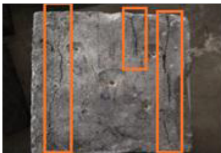
Fig. 2: Initiation of cracks on concrete.
