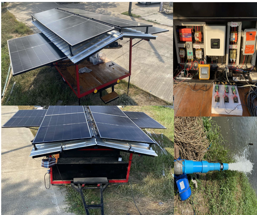
Fig. 1: Real-time operational view of multifunctional and movable solar PV system.
