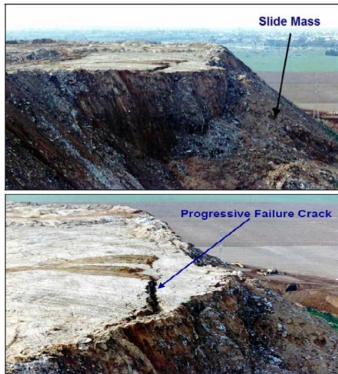
Fig. 2: Failure of Hiriya Landfill (Israel).
