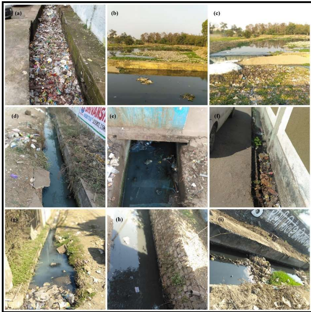
Fig. 2: Informal urban drains choked with solid waste.
