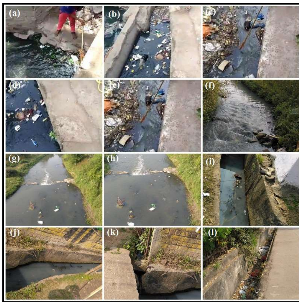
Fig. 1: Different types of informal urban drains carrying liquid waste streams.
