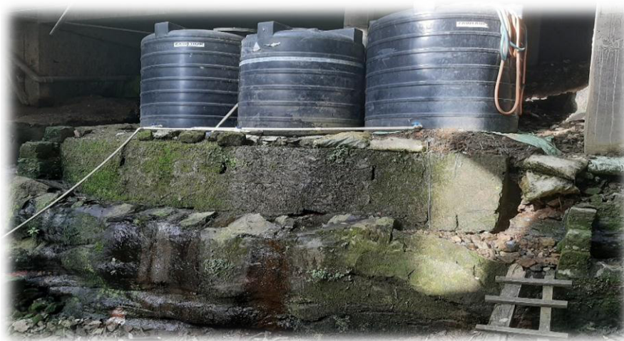
Fig 5: Community rainwater harvesting tanks of Suangpuilawn village.
