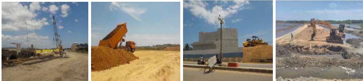
Fig. 2: Activities of land clearing, material transportation, flyover construction, excavation or stockpiling of soil and excavators.
